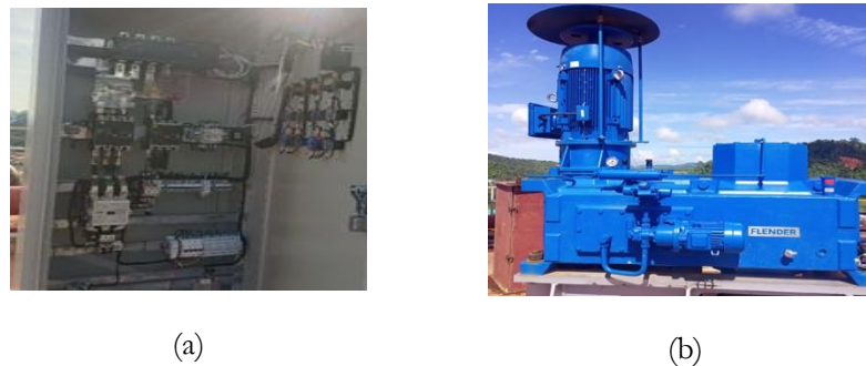
Figure 1. (a) component of electrical control system (b) main drive equipment of agitator.
