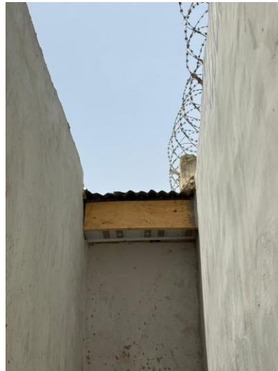
Figure 5. Close-up detail of thin sandcrete block wall and uninsulated corrugated metal roof at a residential building in Katsina, illustrating the absence of thermal barrier between roof and interior
